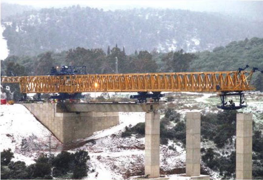
Movable formwork used to install precast segments in span 1 of the Despeñaperros Viaduct. A-4.
